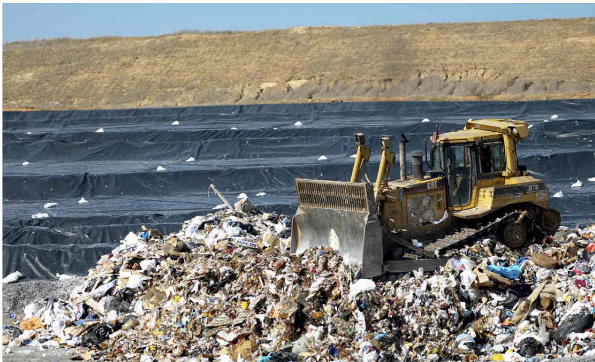
MSW Landfill Active Face; Black Base Liner Appears in Background.
