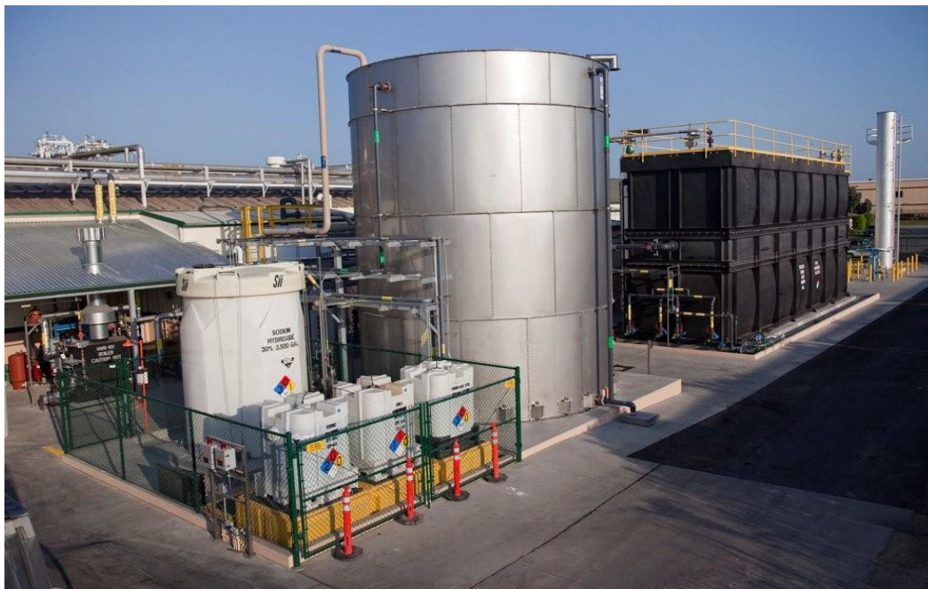
Gill-Onions Anaerobic Digestion Facility; Oxnard, CA
